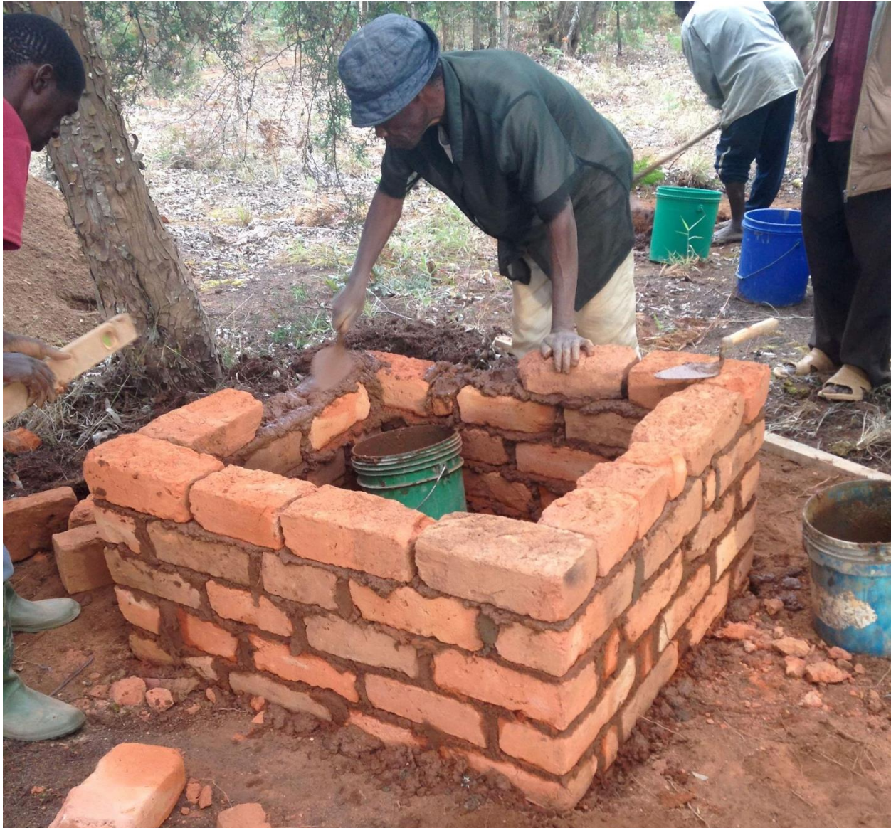
Figure 1: A local builder named Ima constructs the inside of the mud-brick hives
